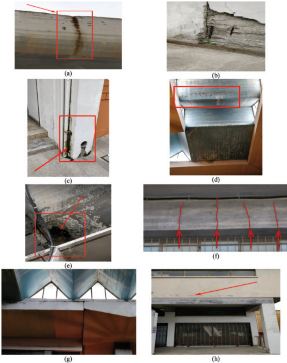
Figure 2. Recorded damages in the old municipal market (2019–2020): (a) Rust stains, (b) Cover delamination and rebar corrosion, (c) Water drainage passing through columns with extensive stains and cracking, (d) Poor cover – exposure of reinforcement – extensive erosion, (e) Mold, stains, efflorescence internally under slab, (f) Deflection cracks on beams, (g) Deformations in the cantilever slab, (h) Horizontal cracks at the connections of the infill walls with the structural system.
