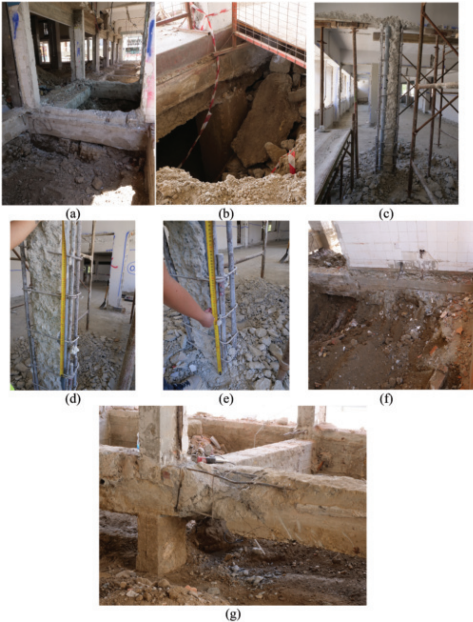
Figure 4. Exploratory excavations and concrete cover removal during retrofit works: (a) lack of foundation slab, (b) holes and ancient ruins under the foundation system, (c) drainage pipes within columns, (d) insufficient stirrup spacing, (e) insufficient lap splice length, (f) lack of foundation of the R/C wall, (g) insufficient flexural and shear reinforcement on foundation beams.
